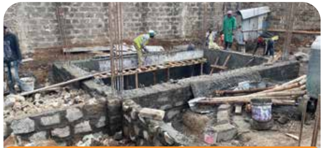
A new residential dwelling in in the course of erection for students who attend the Preca Community in Ruiru, Kenya.
